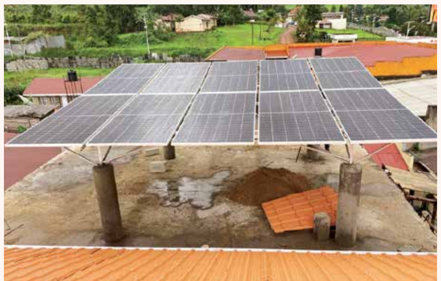
One of the solar panels used at WSACCO
